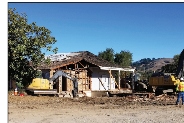
Joaquin Moraga Adobe, built 1841, being restored by Friends of JM Adobe, as a museum.
